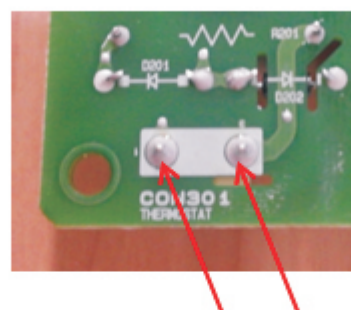
Check CON301 Voltage
