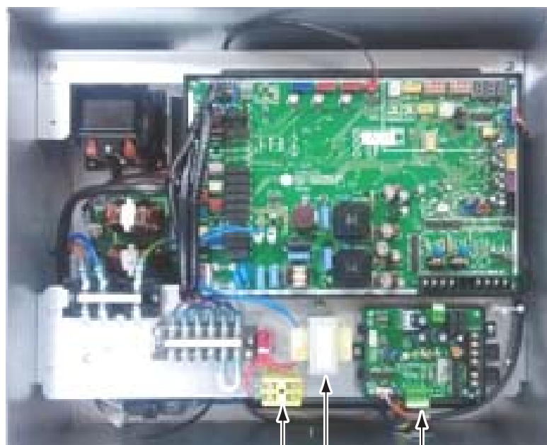
VWFC PCB Transformer Terminal block
