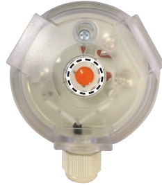
Figure 5 Filter Differential Pressure Switch
